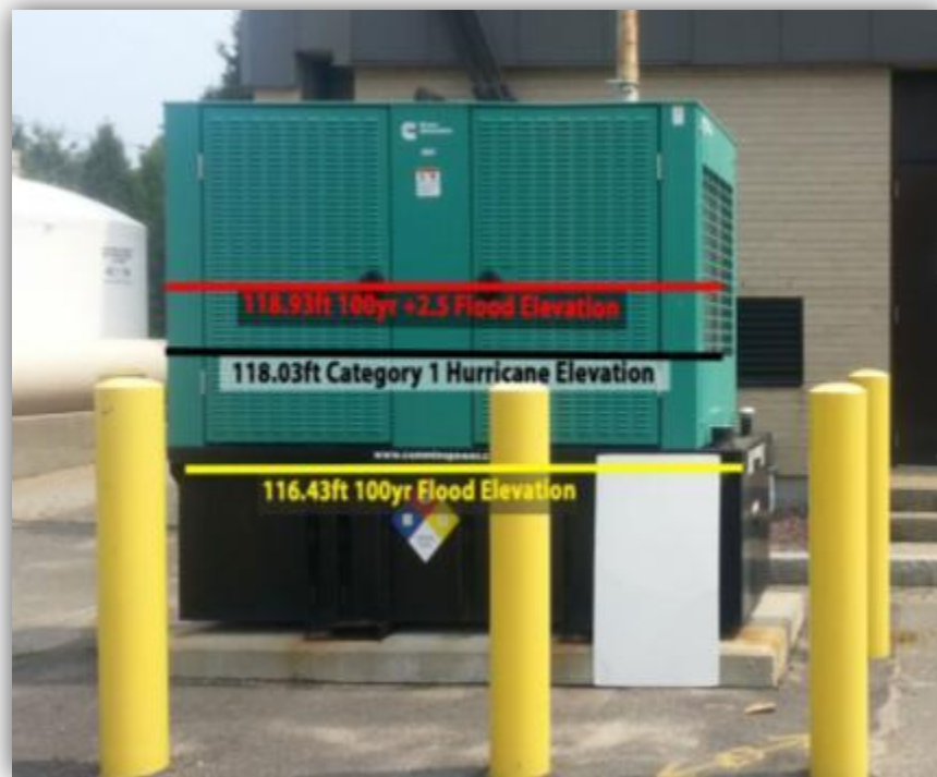
Chelsea Creek Screen House Backup Generator
