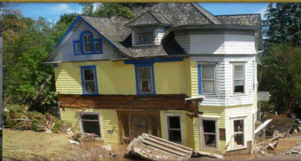
Home washed off its foundation along the Schoharie Creek, Prattsville, NY – Tropical Storm Irene
