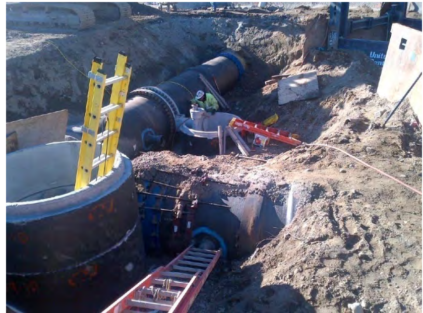
River Road 60-inch WASM 4 Connection
