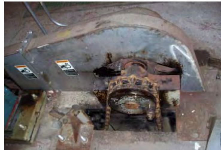
Grit Collector Drive
