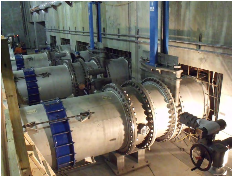
B Side UV Train Installed
