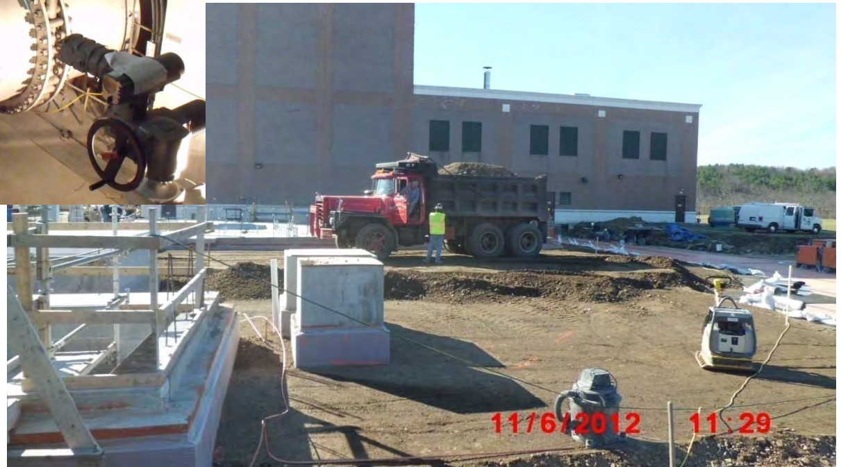
A Side Grounding Rods and Wiring
