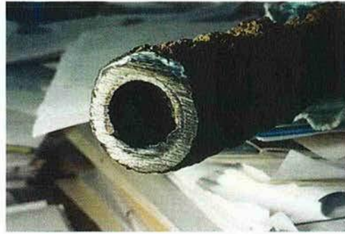
Sample photo of lead-lined service line as found in Quincy
