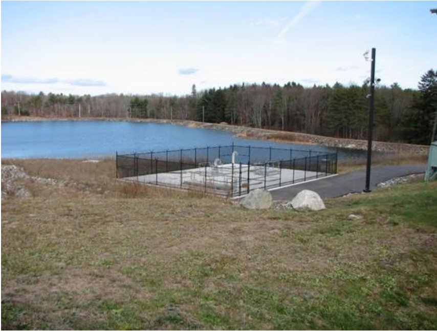
Figure 4.4-3 Valve Chamber - MetroWest Water Supply Tunnel, Weston
