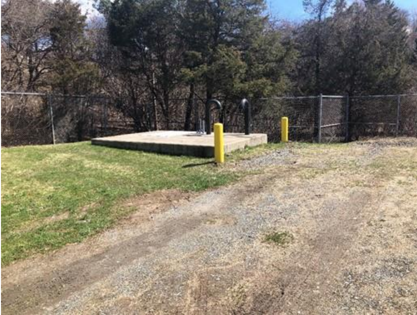
Figure 4.4-5 Top of Shaft and Valve Structure at Connection Site, Metrowest Water Supply Tunnel, Weston
