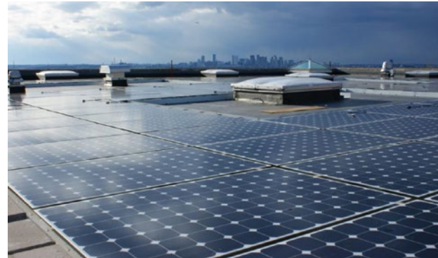
Solar Panels at Deer Island – contribute to renewable energy generated and used on-site.
