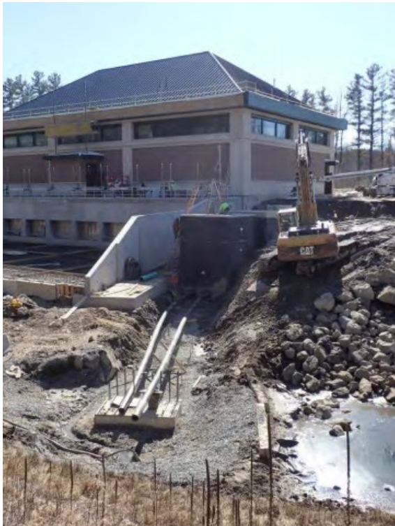
Figure 8: WAPS Geothermal Heat Pump and Solar Power Installation
