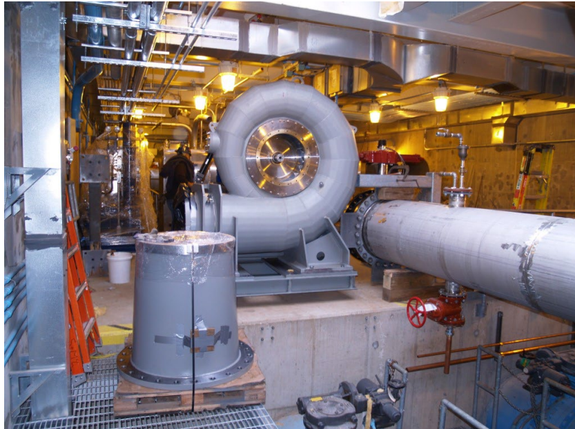
Figure 2: Loring Road Hydroelectric Turbine Generator during construction. This turbine generates on average 1.2 million kilowatt hours per year.
