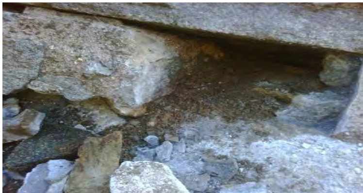
Major voids in upstream side of Quabbin spillway
