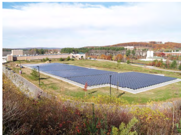
476 kW photovoltaic system at Carroll
