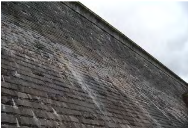
PCB-contaminated efflorescence and mortar
