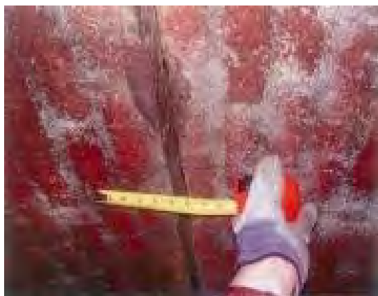
Crack in Crown of Pipe
