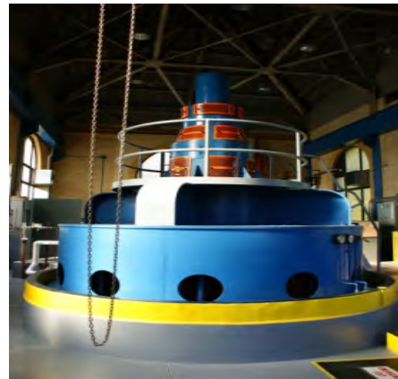
Hydro Turbine at Oakdale
