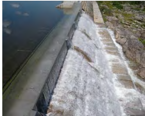
Stainless steel mechanical crest gate, new sill at 390' BCB
