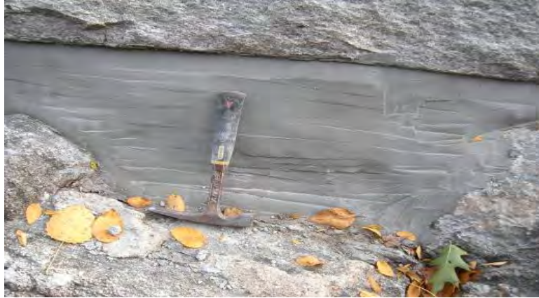
Major voids repaired, injection-grouted and mortared
