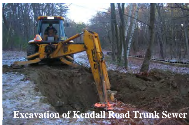
Failed Trunk Sewer off Kendall Road
