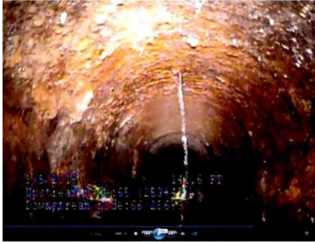
Infiltration Entering Trunk Sewer
