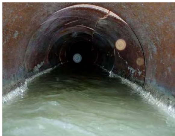
Example of sewer needing rehabilitation
