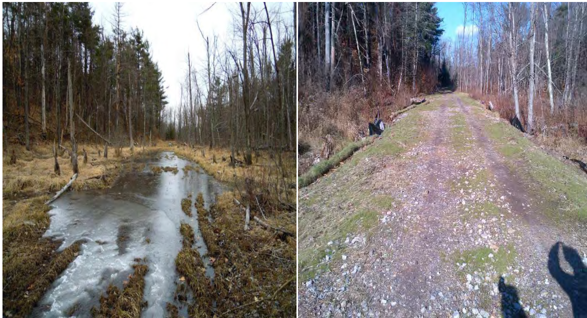
Photos above show before and after repair of flooded RHS easement MH 6A – MH 10
