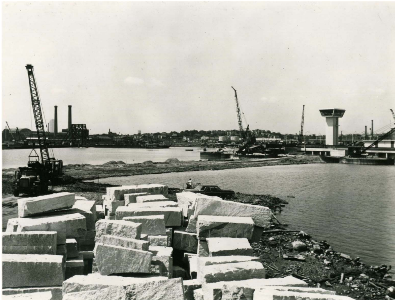
Metropolitan District Commission Mystic River Basin Elevation Control Project Everett-Somerville, Mass. MDC Contract 1360 General view from Everett side.
